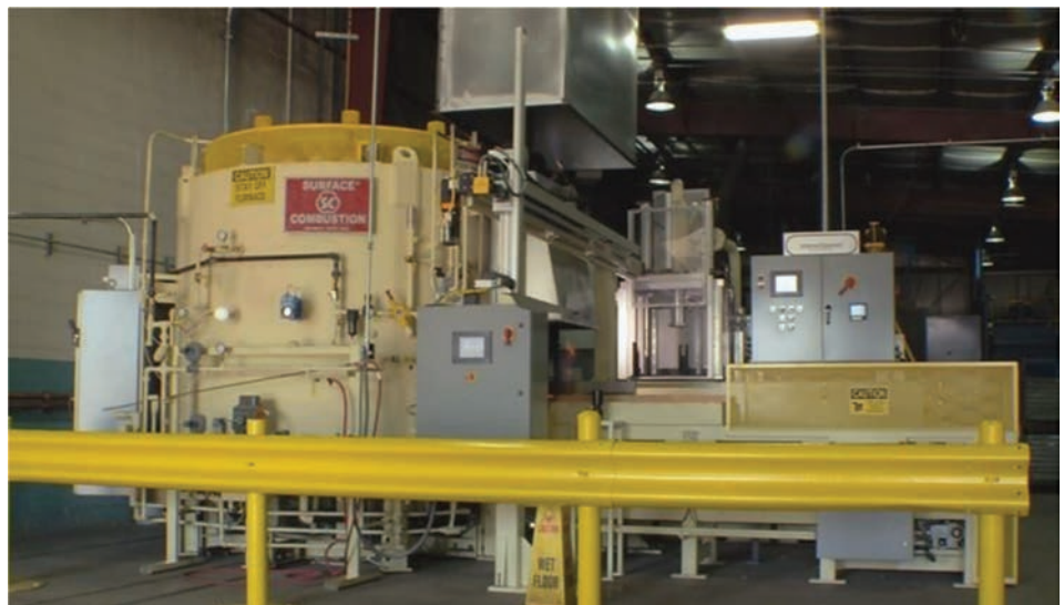
Fig. 23 Fully automated single-part processing IQ-3 system equipped with a controlled atmosphere rotary hearth furnace, pick-and-place device part transfer automation, and a water quenchant chiller
