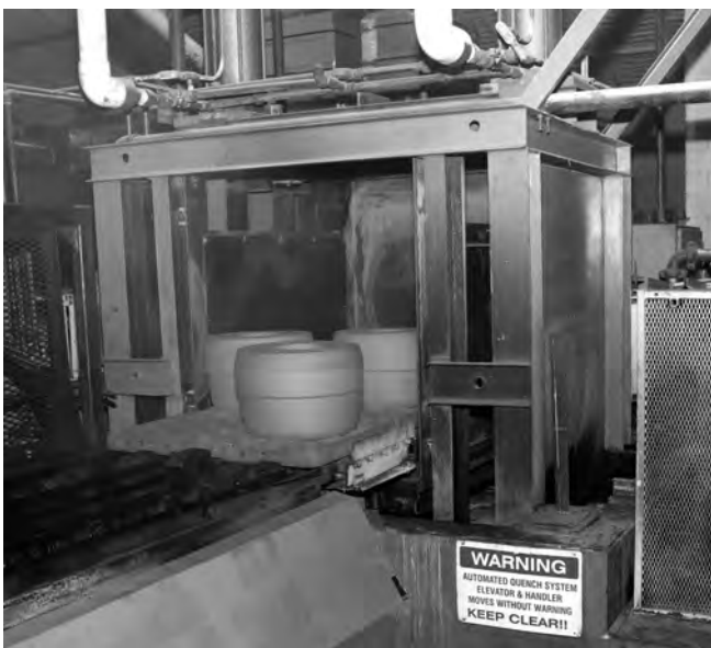
Fig. 15 Batch-type intensive quenching (IQ) system with stand-alone IQ water tank. Courtesy, Akron Steel Heat Treating Co.
